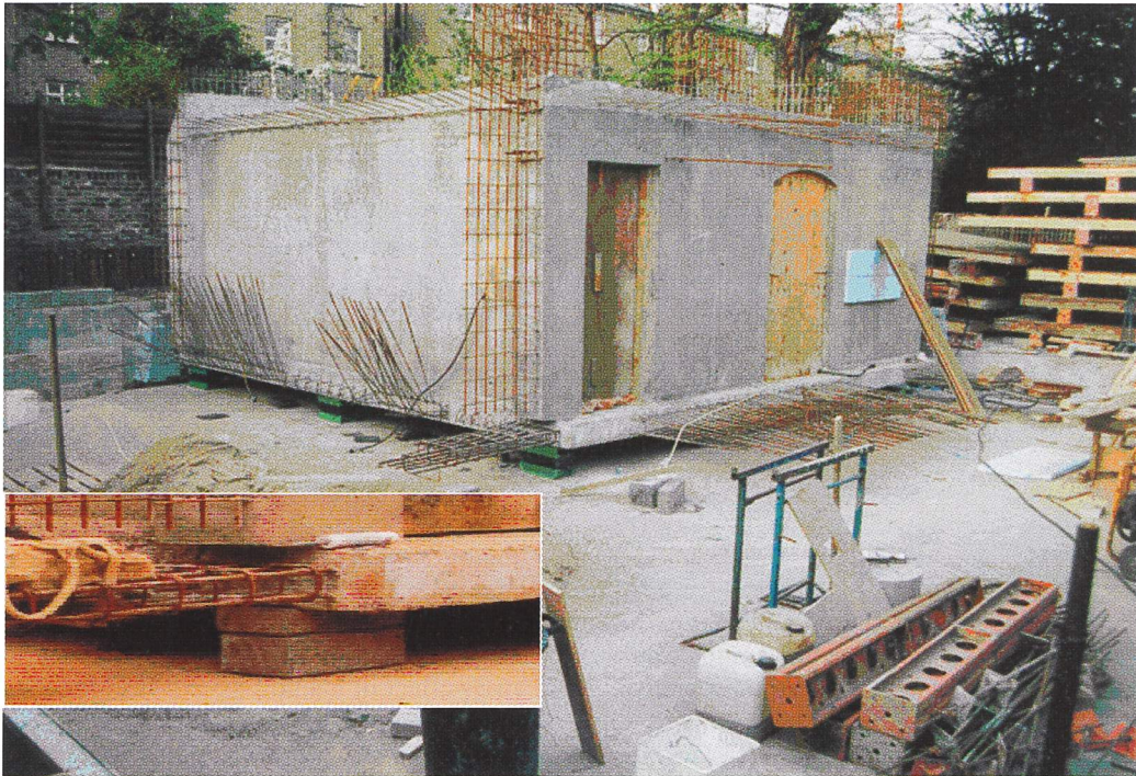
Figure 2 Test Room on GERB Coil Springs, Test Room on Blocks (Inset)
