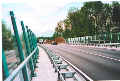
Acoustic barriers restrict noise propagation
